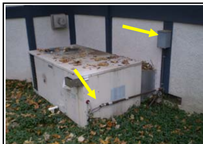
Left side unit gas shut-off & AC disconnect.
