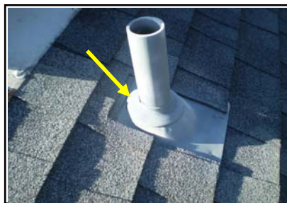
Cracked weather collars may allow water entry into attic.
