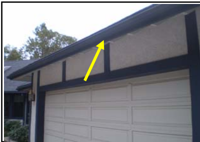
Leaking noted at multiple gutter joints.
