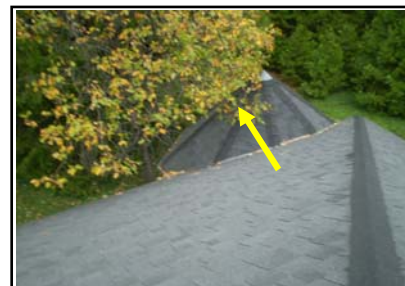
Recommend keeping vegetation trimmed off & away from roofing.
