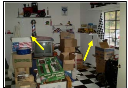
Open ground wiring noted at storage room wall outlets.
