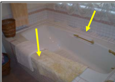
Master bathroom - recommend regular tile sealant application.
