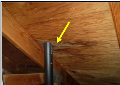
Staining noted at vent pipe entry through roofing.
