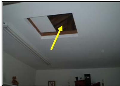
Attic access opening reduces garage to house fire protection.
