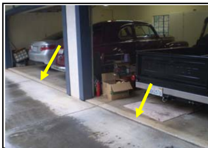
High edges noted across garage entry.
