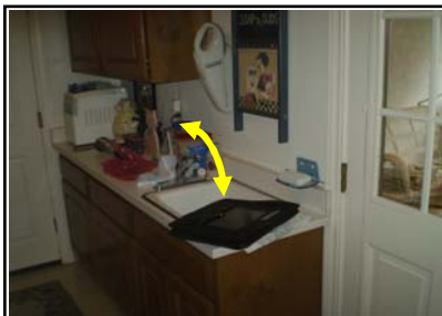
Sink counter outlet is not GFCI protected - recommended.
