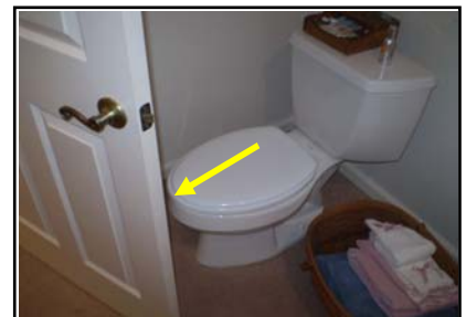
Bathroom door opens against toilet.
