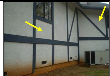
Recommend sealing cracks in stucco surfaces.
