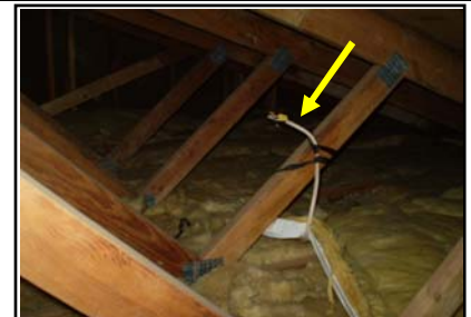
Exposed wiring noted in right rear attic.
