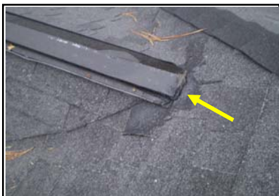
Recommend replacing worn & cracked sealant.
