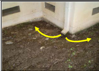
Downspout are discharging run-off against house.
