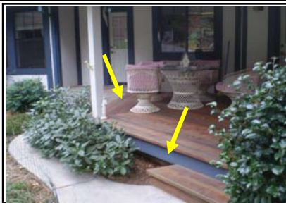
High edges noted off front decking.
