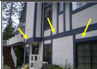
Worn & missing caulking noted along trim seams & edges.
