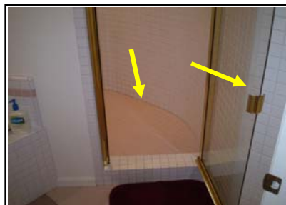
Shower door opens against wall. Keep seams & edges sealed.
