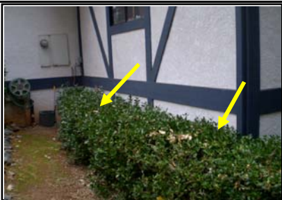
Recommend keeping vegetation trimmed away from siding.
