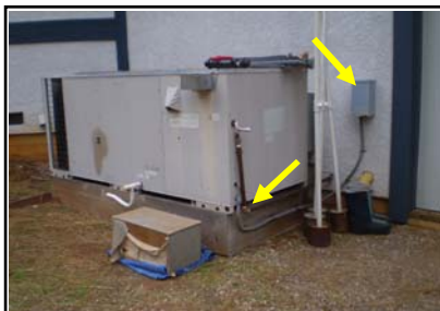
Right side unit gas shut-off & AC disconnect.
