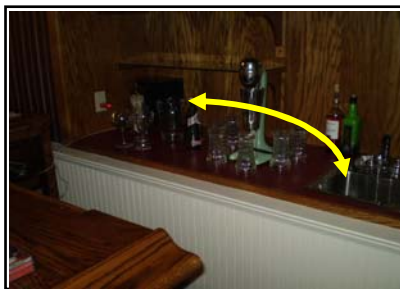
Wet bar counter outlet is not GFCI protected - recommended.
