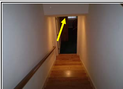
Low head clearance noted down stairs.
