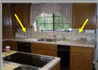
Kitchen counter outlets are not GFCI protected - recommended.
