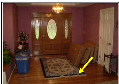
Front entry shading noted to flooring at area rug.
