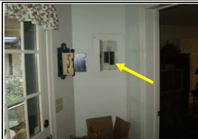
Sub panel is located in laundry area.
