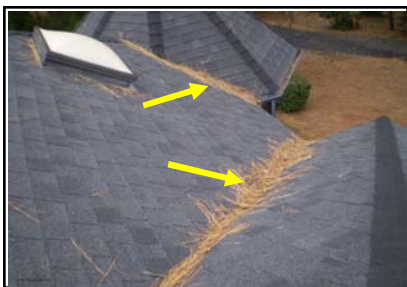
Recommend keeping debris cleared from roof valleys.
