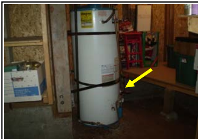
WH # 1 - older unit. SRV is not drained to building exterior.
