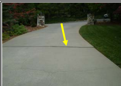
Uplifting edge noted at driveway.
