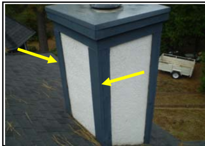
Recommend keeping chimney chase exterior caulked/ sealed.
