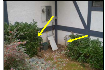
House main gas & water shut-off valves.
