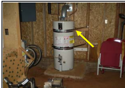
WH # 2 - newer unit. SRV is not drained to building exterior.
