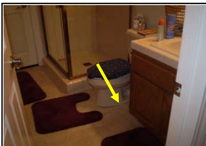
Bathroom # 3 - toilet is not secured to floor.
