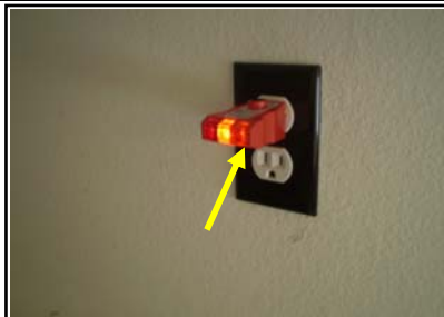
Open ground wiring noted at garage storage room outlets.
