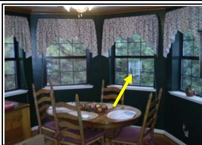
Failing thermo seal noted in eating nook window.
