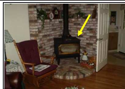
Unable to verify wood stove clearance recommendations.
