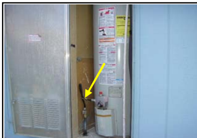
Water heater gas shut-off valve.
