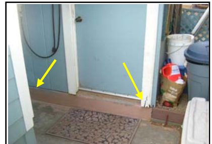
Deterioration noted to shed exterior siding & trim.
