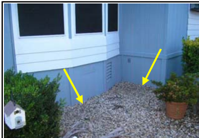
Earth to wood contact to wood skirting.
