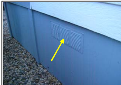
Recommend replacing louvered covers with open mesh screens.
