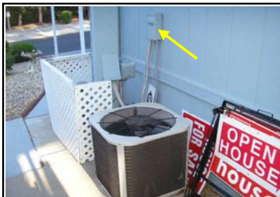
AC condenser & disconnect.
