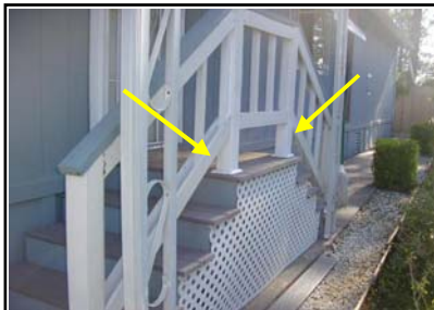
Deterioration noted to side entry railing material.
