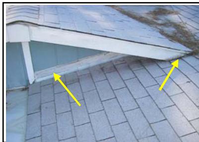
Deterioration noted to front siding trim & fascia material.
