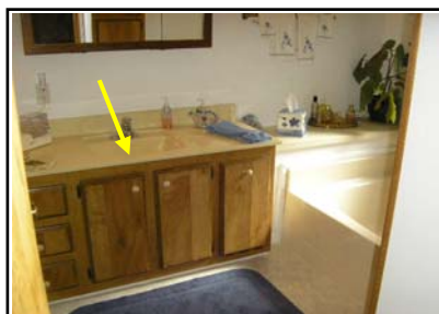
Master bathroom - sink overflow drain not draining.
