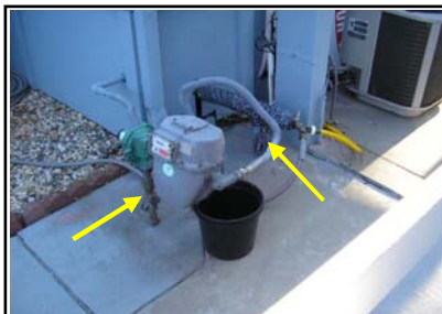
Main gas shut-off - left. Water shut-off valve - right.
