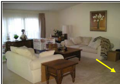
Living room - loose & squeaking sub floor noted.
