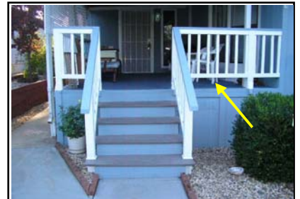
Openings under railings exceed 4 " recommended maximum.
