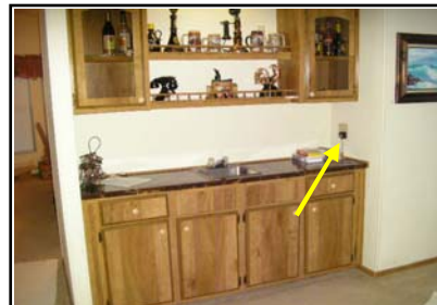
Recommend upgrading sink outlet to GFCI.
