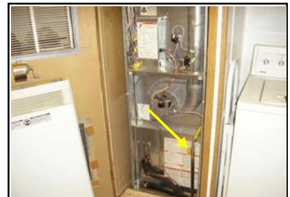
Furnace gas shut-off valve located behind bottom panel.
