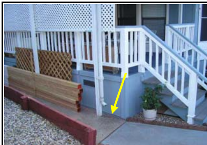
Front deck - earth to wood contact noted.
