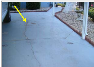
Cracking & uplifting noted to driveway material.
