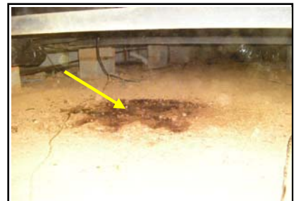
Leaking noted under bathroom # 2.
