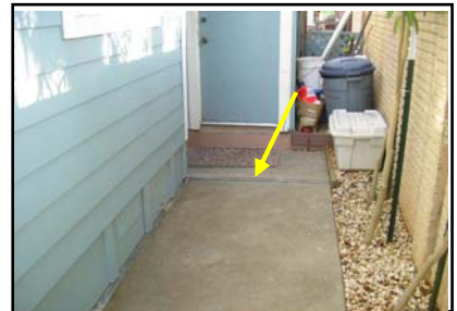
Uplifted edge noted along rear walk.
