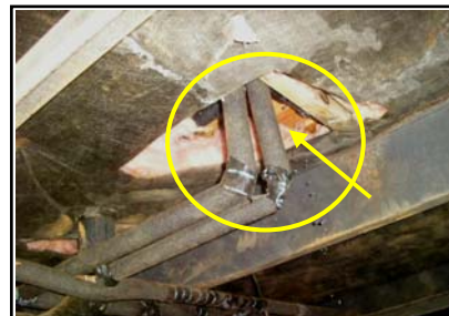
Leaking noted under bathroom # 2.
