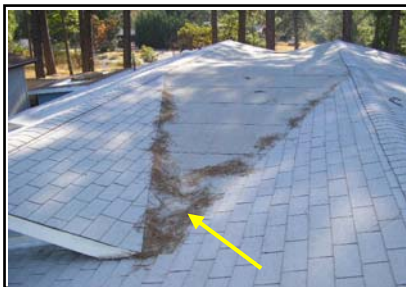
Debris noted on rolled comp roofing surface.
